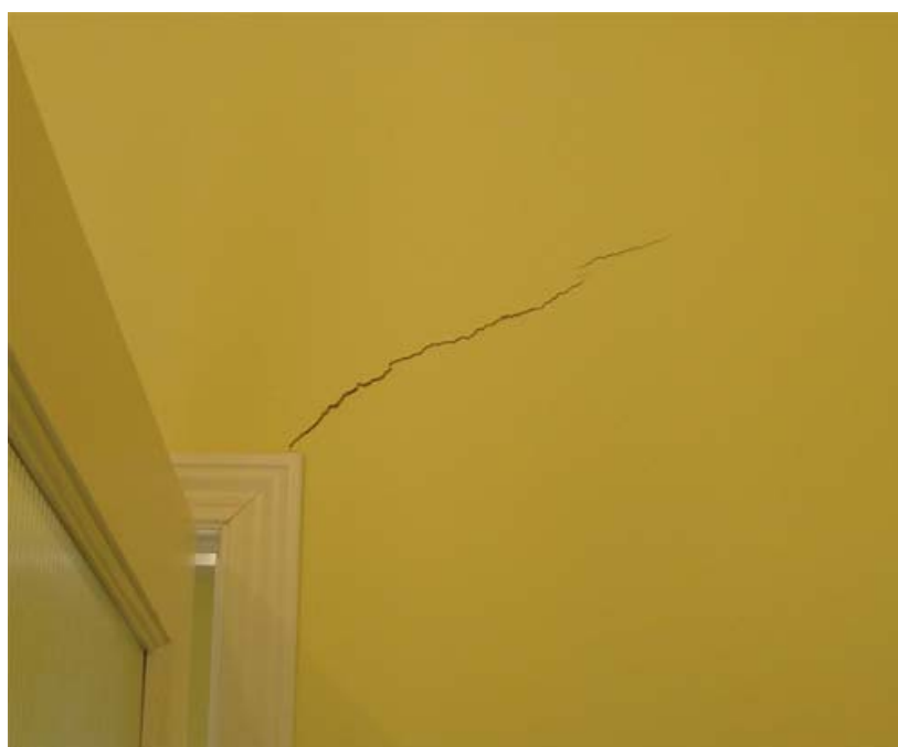
Typical drywall crack
